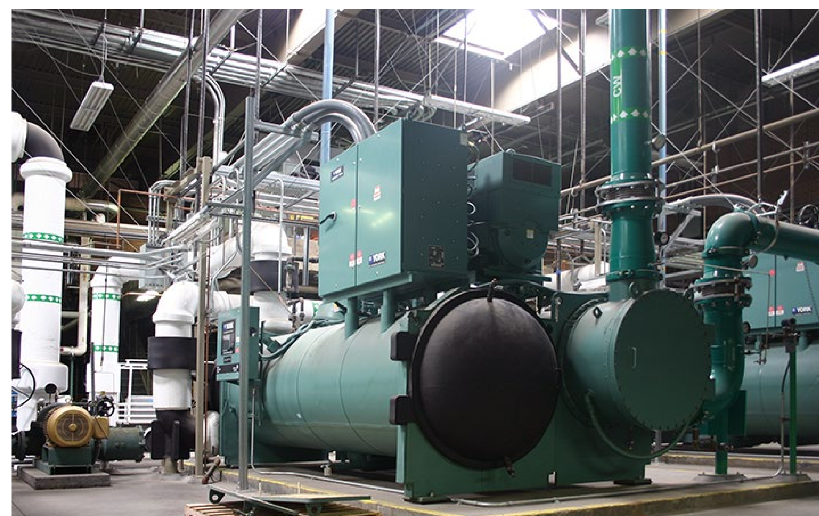
Figure 3: Photo of San Jose State University's advanced variable-speed chiller within the Central Utilities Plant. [3]
